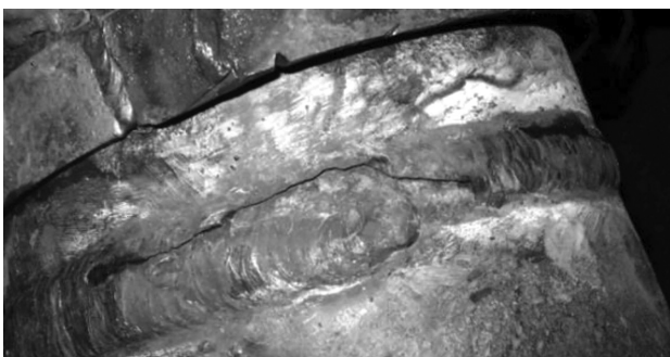
Figure 5: Crack near weld on the superheater-P2 collector metallurgical analysis Slika 5: Razpoka blizu zvara na pregrevalniku P2 metalurška analiza zbiralnika
